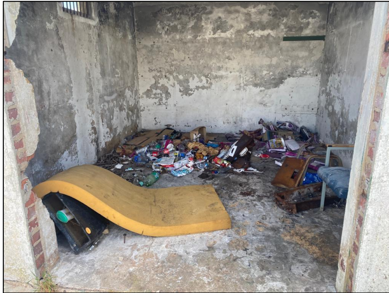
Figure 7. Unsecured waste at Signal School.
